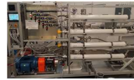
Pilot-scale Water Reuse System
